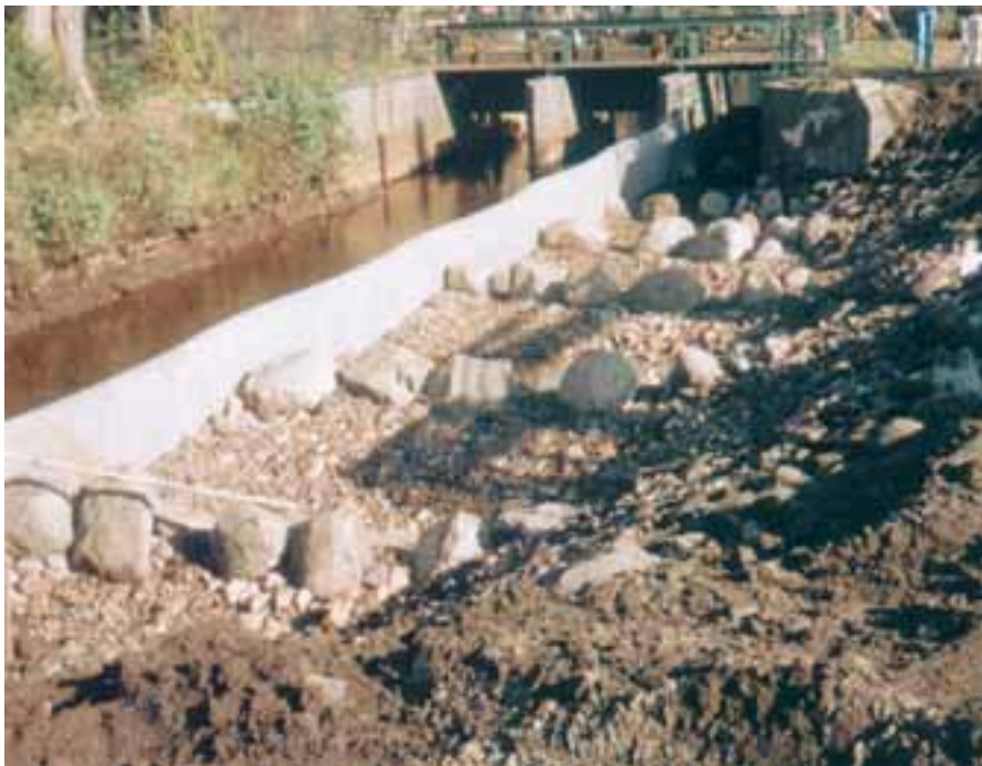
Figure 4.36: Delmenhorst fish ramp.
